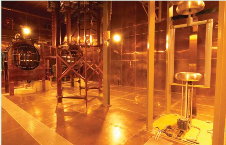
Converter room: large variable coil for impedance matching (left), large fixed coil (center), and drive unit for connecting the antenna to the earth (right)
