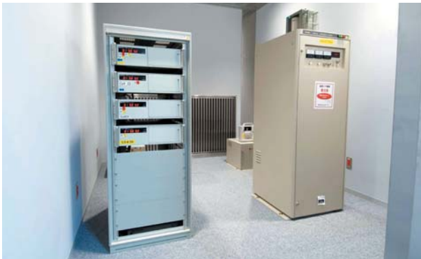
Figure 2: Four cesium atomic clocks (in the rack on the left) and a hydrogen maser frequency standard (on the right) installed in shielded Room 3
