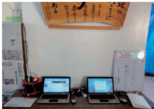
Figure 3●Internet access via a cognitive wireless router set up in evacuation center at elementary school
