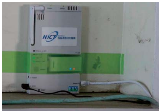
Figure 2●Cognitive wireless router providing Internet access
