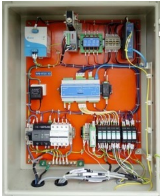
RTU module installed in RTU box
