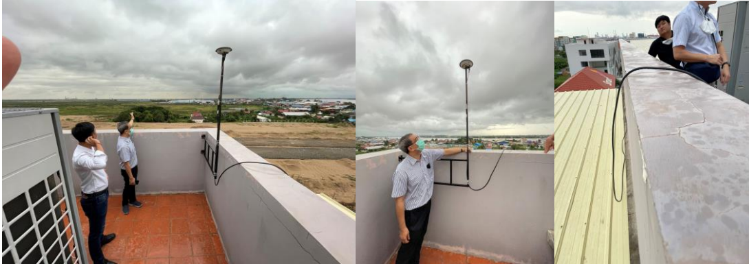
Fig. 4. Checking the GNSS antenna and its cable installation at the rooftop of the CADT -Innovation Center.
