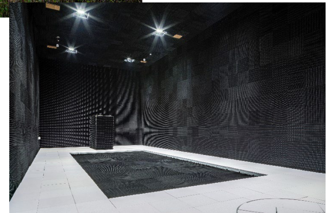
B5G anechoic chamber
