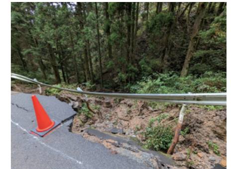
Figure 5 Hagane-yama Transmission Station Road cave-in caused by typhoon
