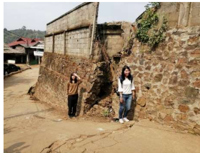
Site of crack in the ground
