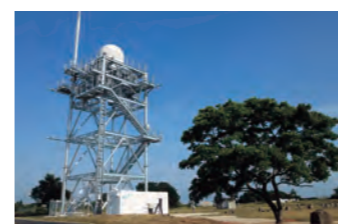
PANDA tower and container installed at the Advanced ICT Research Institute
