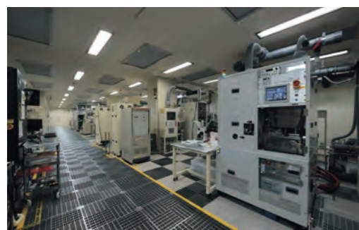
Processing equipments in the clean room
